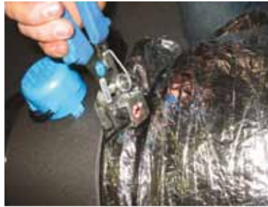
Air Condition Duct
